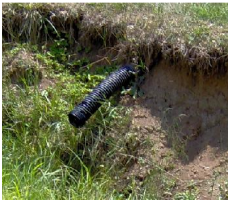
Figure 17: Pipe Entering Stream
